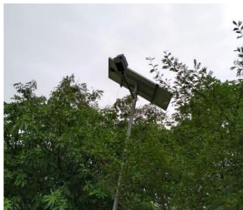
Solar Lights installed
