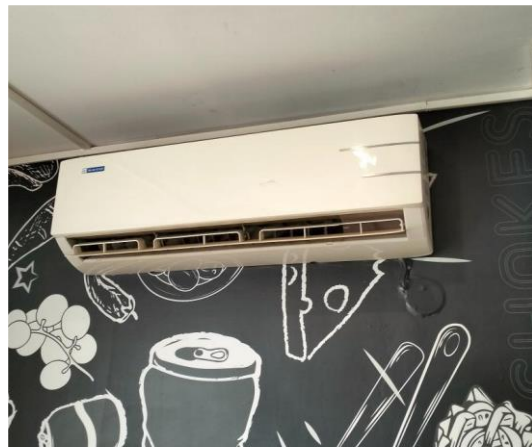
Split AC Installed
