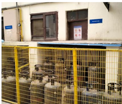
LPG cylinders placement
