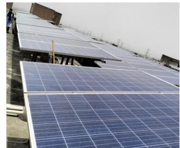
Solar PV installed on building roof
