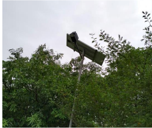
Solar lights installed
