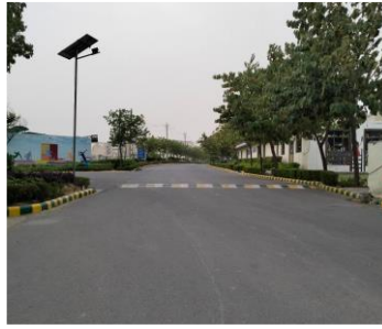
Solar lights installed
