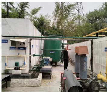
STP plant to treat wastewater
