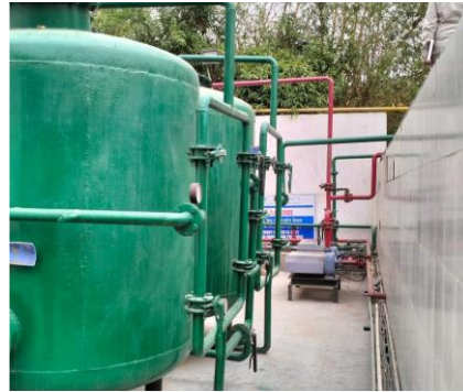
STP installed (250 KLD)
