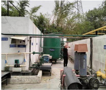
STP installed (250 KLD)
