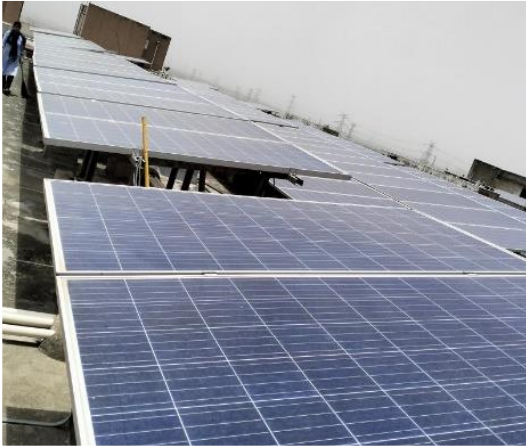
Solar Panel Installed
